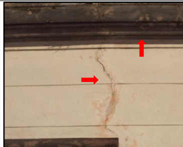
Fissura Vertical; Bolor.
